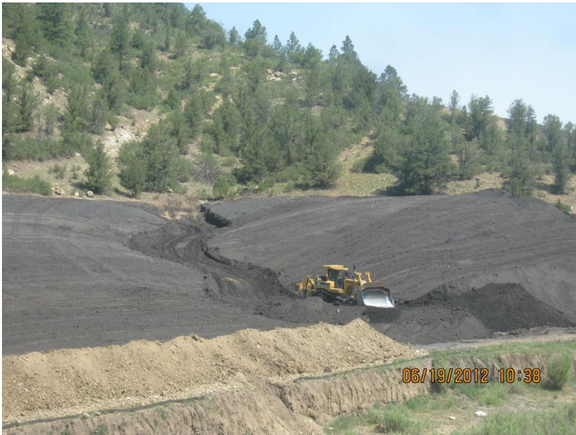
Figure 18. Embankment preventing coal waste fill within the meander belt of the restored channel.
