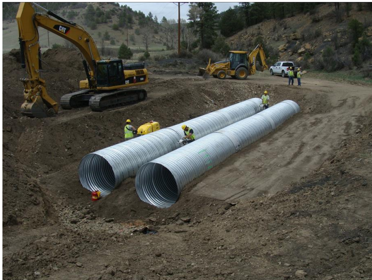
Figure 12. Culverts that convey the Coal Canyon channel under the realigned road.
