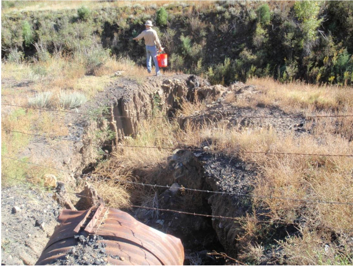
Figure 23. Culvert conveying outflow from the wildlife ponds to the Dutchman Canyon channel.
